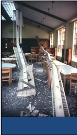
1983 Coalinga, CA Earthquake
